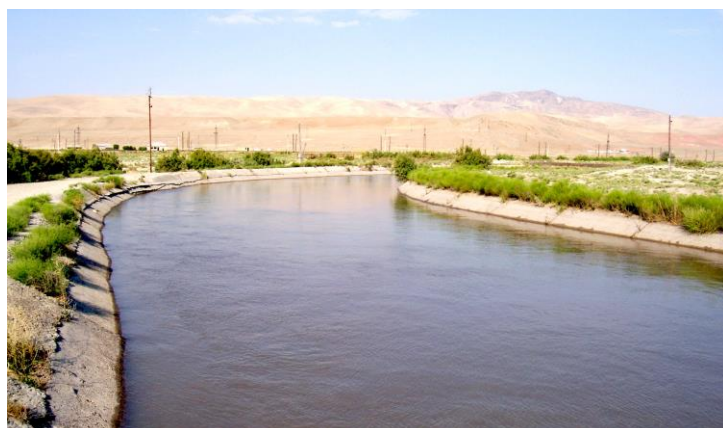
Fig 1: General view of the Samur-Absheron Canal. There are concrete slabs covering the bottom of this watercourse
