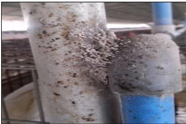
Fig 1: Mites with dust on the water and drainage pipelines
